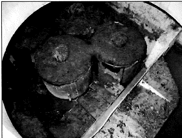
Media Cartridge Filter Vault with Accumulated Sediment
