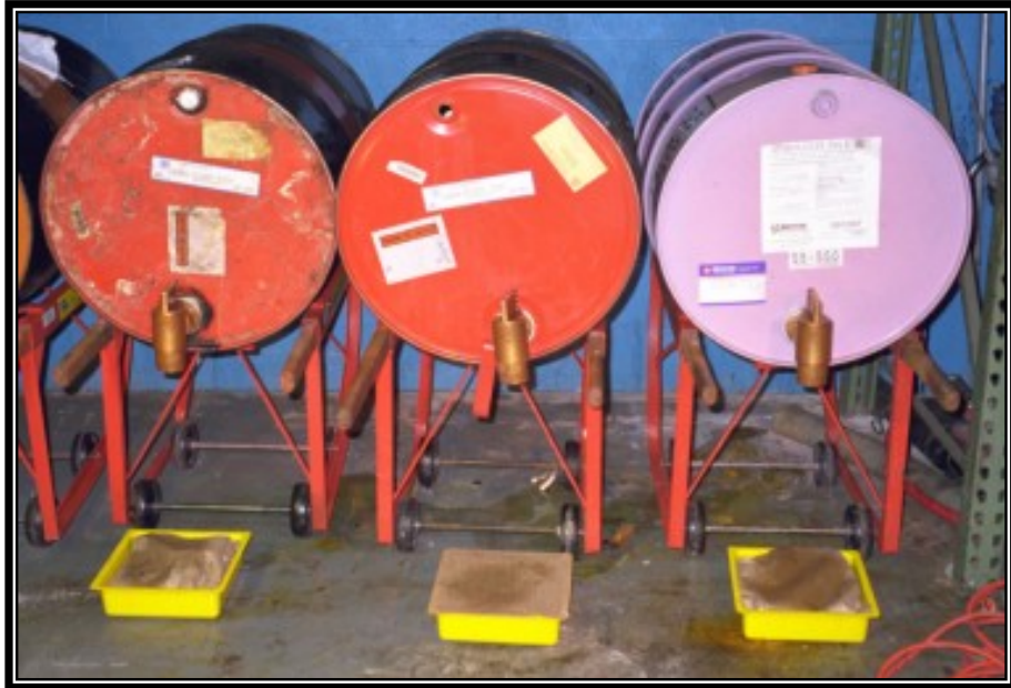
Figure 4.18. Mounted Containers with Drip Pans.
