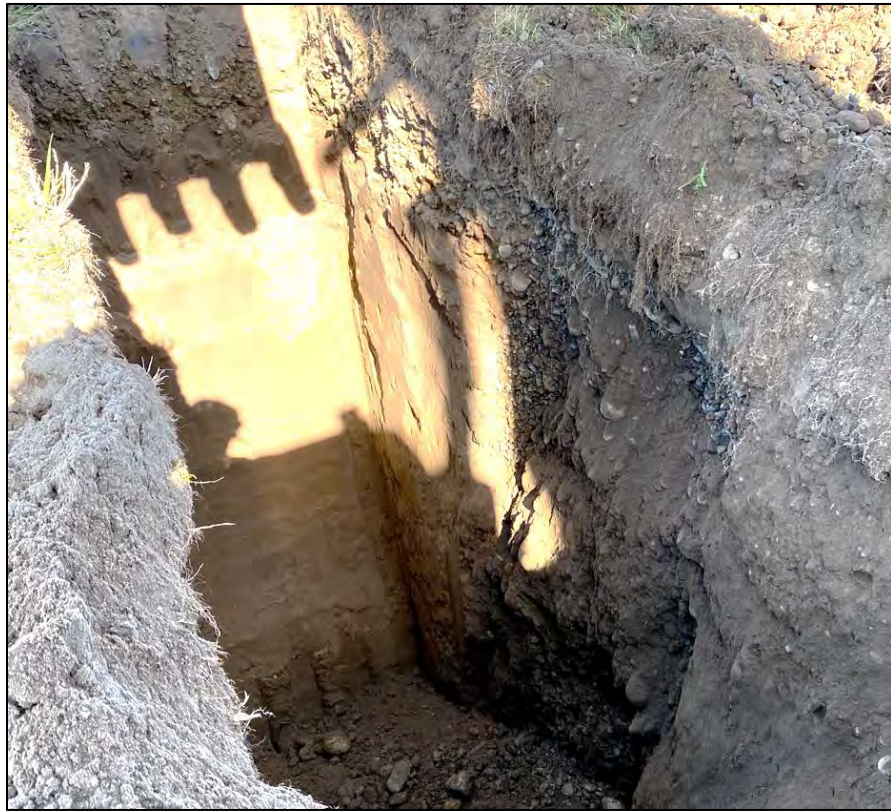
Plate 1. View of TP-3. Caving of gravel column seen in pit sidewall.
