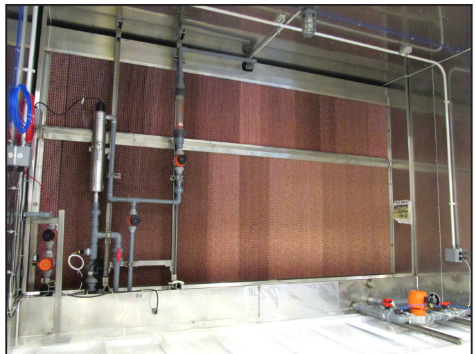
Evaporative Cooler Air Leaving Side
