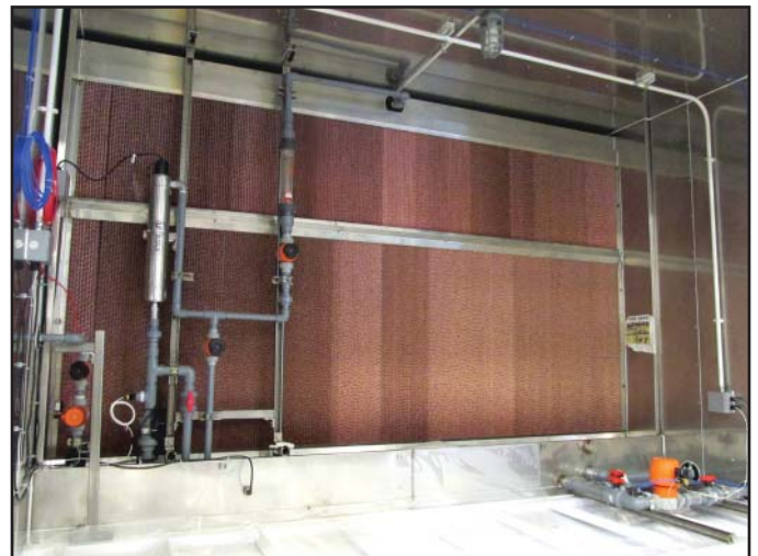
Evaporative Cooler Air Leaving Side
