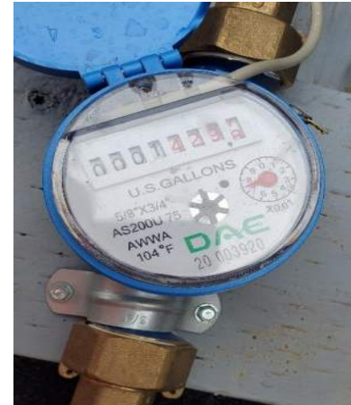
1-hour GPM Test
