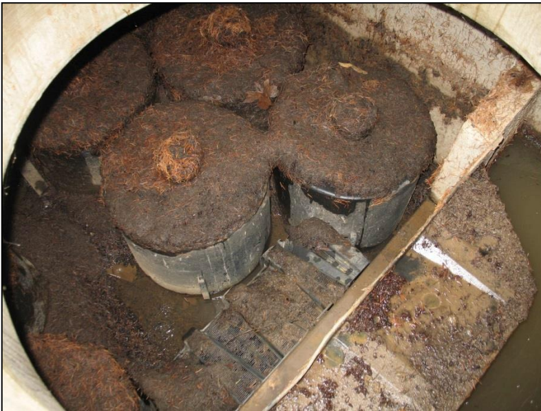
Media Cartridge Filter Vault with Accumulated Sediment
