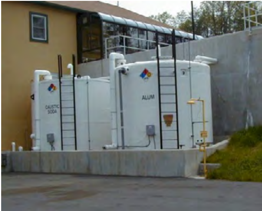
Figure 4.19. - Aboveground Storage Tanks with Secondary Containment.
