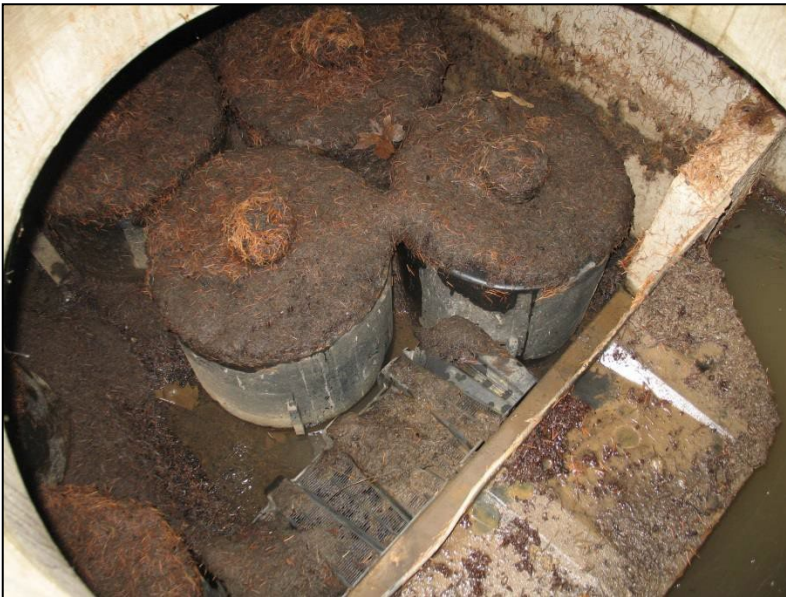
Media Cartridge Filter Vault with Accumulated Sediment
