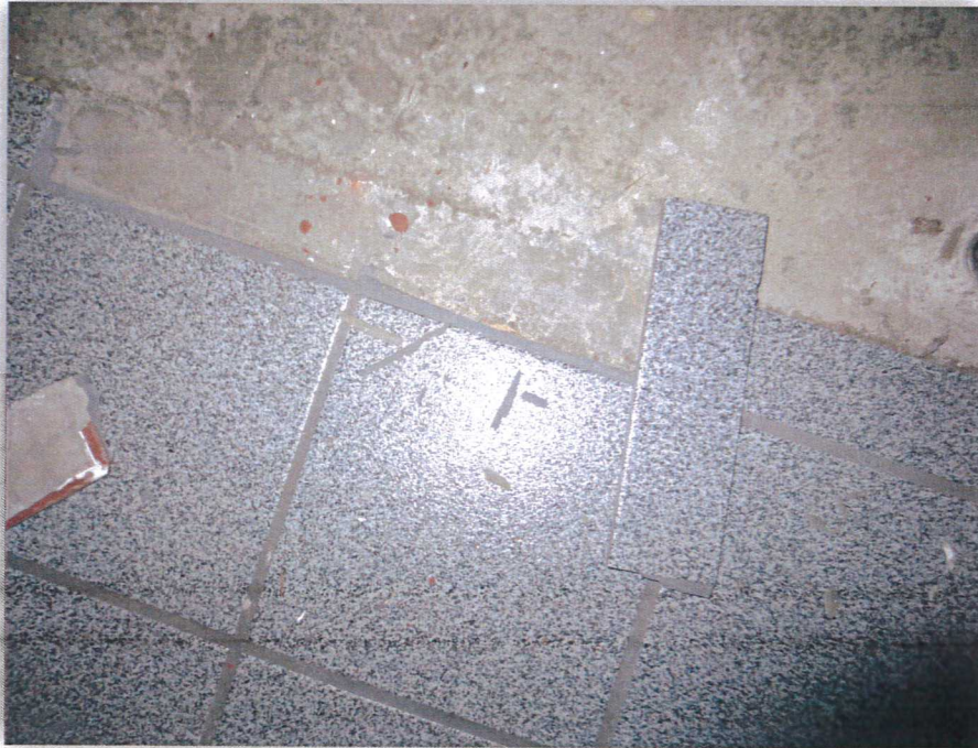
Photo 41: Ceramic Tile Grout
