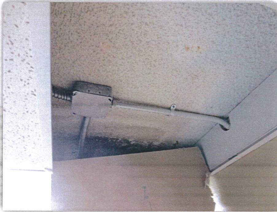
Photo 23: Popcorn Ceiling Texture
