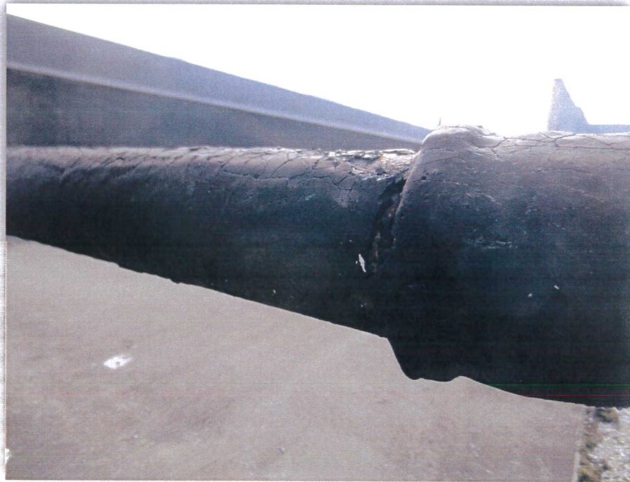
Photo 32: Tar on Piping
