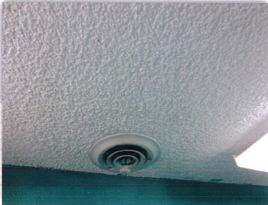
Photo 24: Popcorn Ceiling Texture
