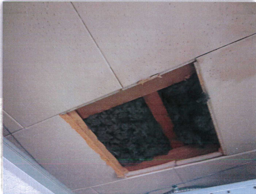
Photo 22: White Stapled on 12x12 Ceiling Tile
