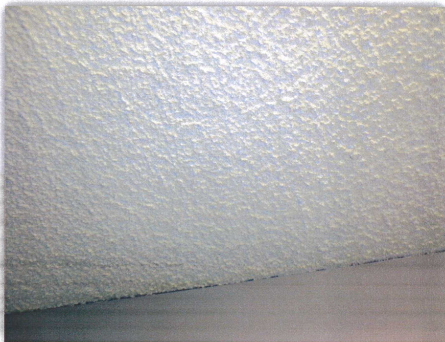
Photo 25: Popcorn Ceiling Texture
