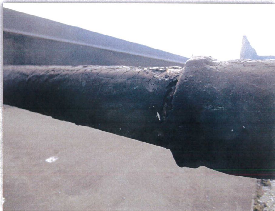
Photo 32: Tar on Piping
