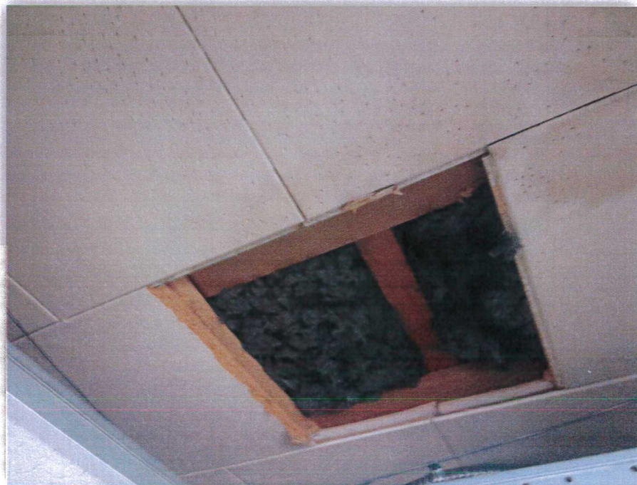
Photo 22: White Stapled on 12x12 Ceiling Tile
