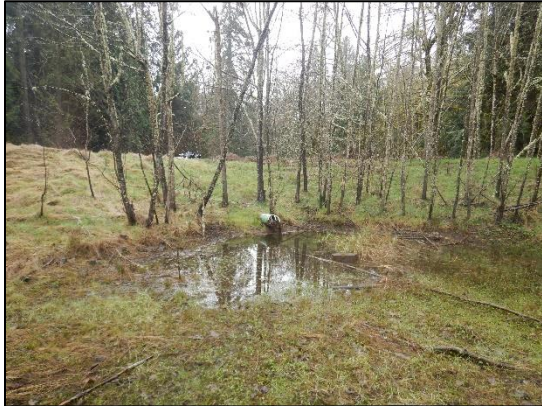
Figure 2. Stormwater Pond Conveyance Features
