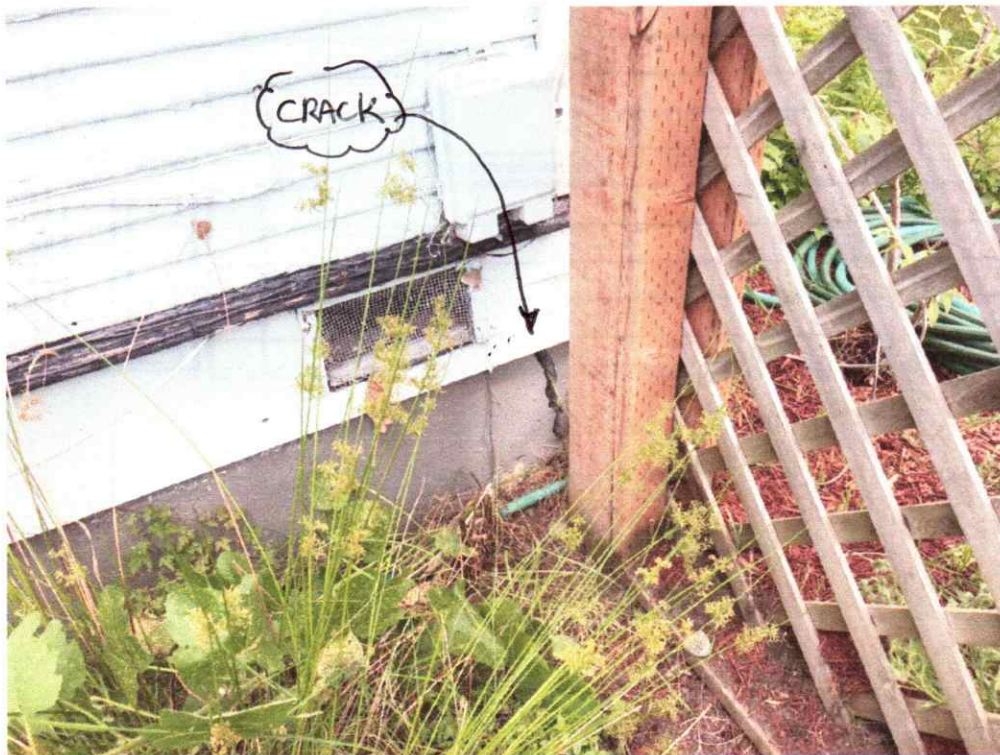
Cracked Foundation at the Southeast Corner - Two Piers and Angles under this Corner
