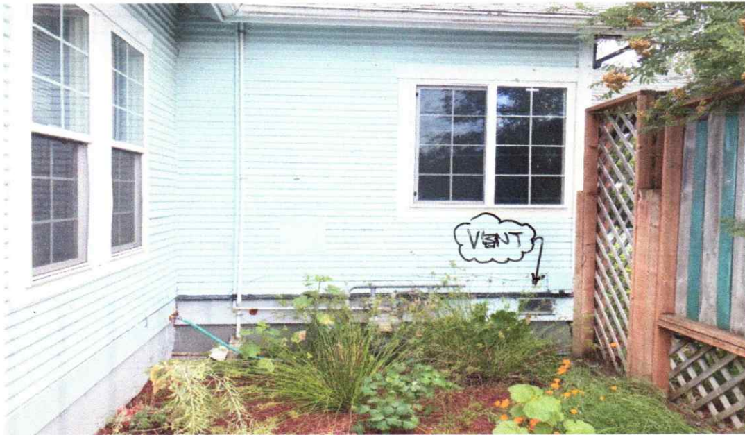
View from South looking at the South Wall – Add Pier near Vent Hole
