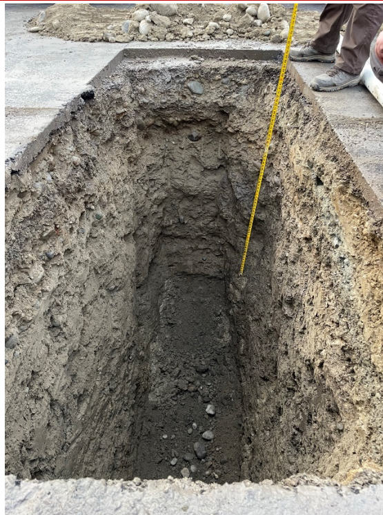
Photo 2: Temporary Water Seepage at PIT-01
