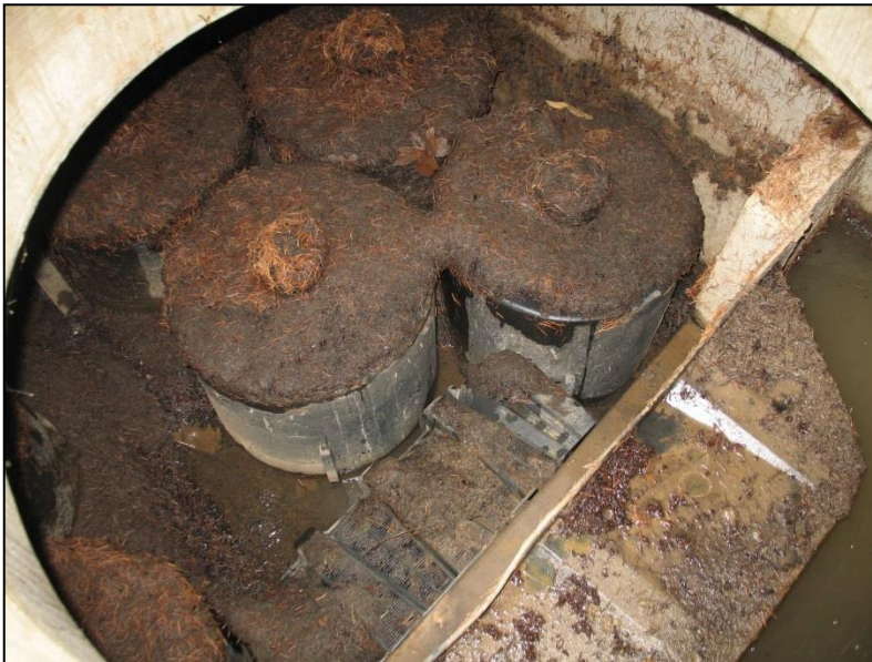
Media Cartridge Filter Vault with Accumulated Sediment
