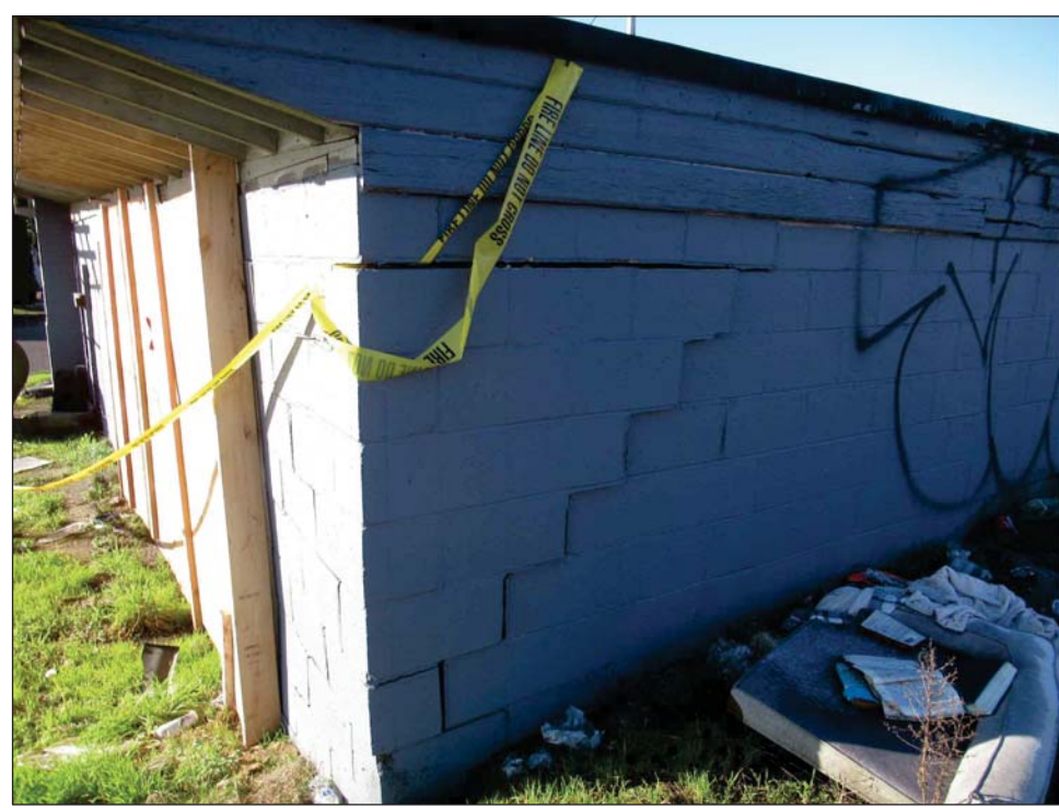
NORTHEAST CORNER OF DAMAGED CMU WALL
