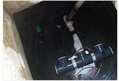
Manifold Tee View of a Cleaned System
