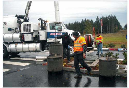
BayFilter System Cleanout
