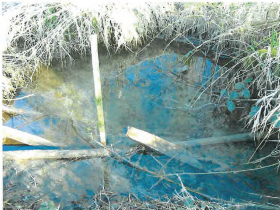
Photo #14: Looking down at what appears to be the inlet end of an old buried drain pipe (see Figure 7) that is flowing under head pressure due to water level in pool (noted small whorl pool in water >2' deep). (IMG-037, 3/4/20)
