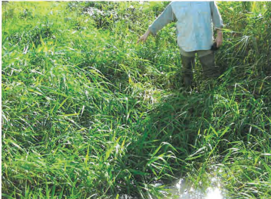
Photo #5: Looking directly down into the small, overgrown drainage ditch just east of the property line. The location of this portion of the ditch is near the central part of this property. Note the slow flow out of this area is due to clogging by dense vegetation (Reed Canary Grass). (Taken 9/28/07)
