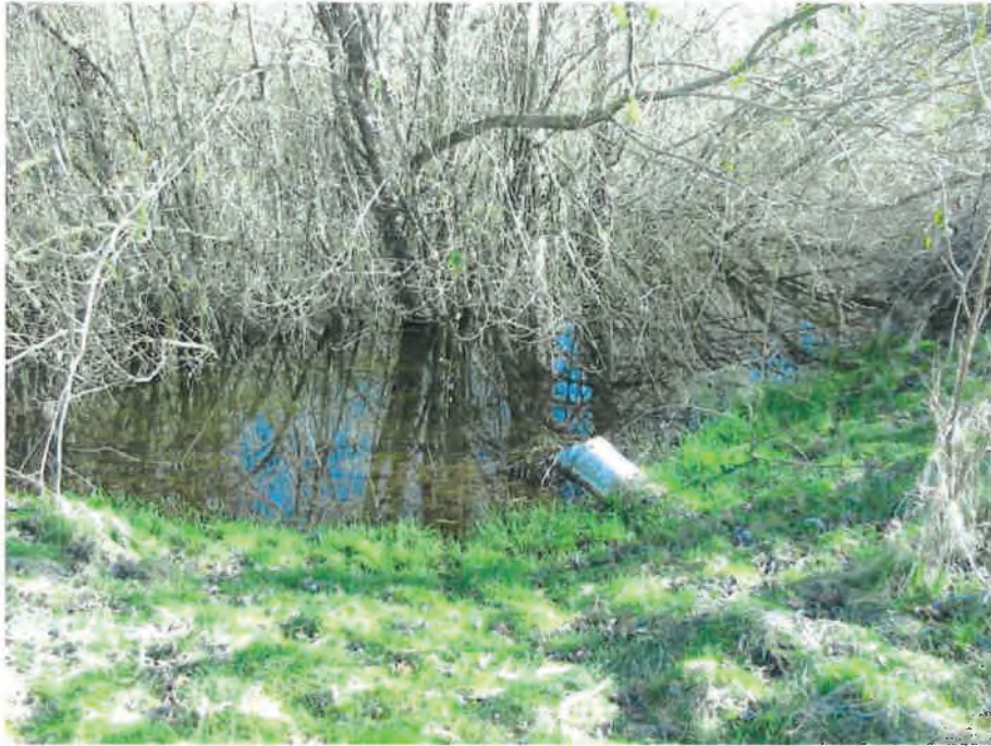
Photo #13: Looking down at the 12" CMP outlet from the storm water detention pond that is constructed in the surveyed location shown on Figure 7. Note the standing water is actually flowing out at this time due to the diverted stream flow into the pond. (IMG-033, 3/4/20)
