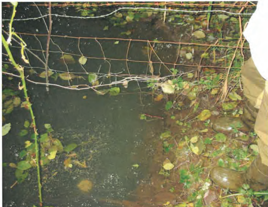
Photo #8: Looking directly down at the submerged end of the culvert that is located directly beneath the flag shown in Photo #7. At this time the water is flowing slowly north in the ditch and into the upstream end of the culvert. This area requires maintenance and possibly a larger culvert. (Taken 9/28/07)
