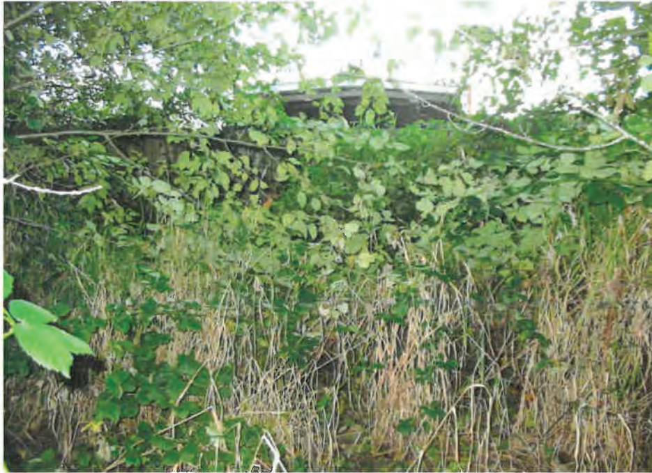
Photo #9: Looking west from the same location as at Photo #8 about 30 ft. south of the southeast property corner. Notice the dense vegetation (reed canary grass, Himalayan blackberries and red alder trees overgrowing the ditch and culvert pipe in this area. (Taken 9/28/07)
