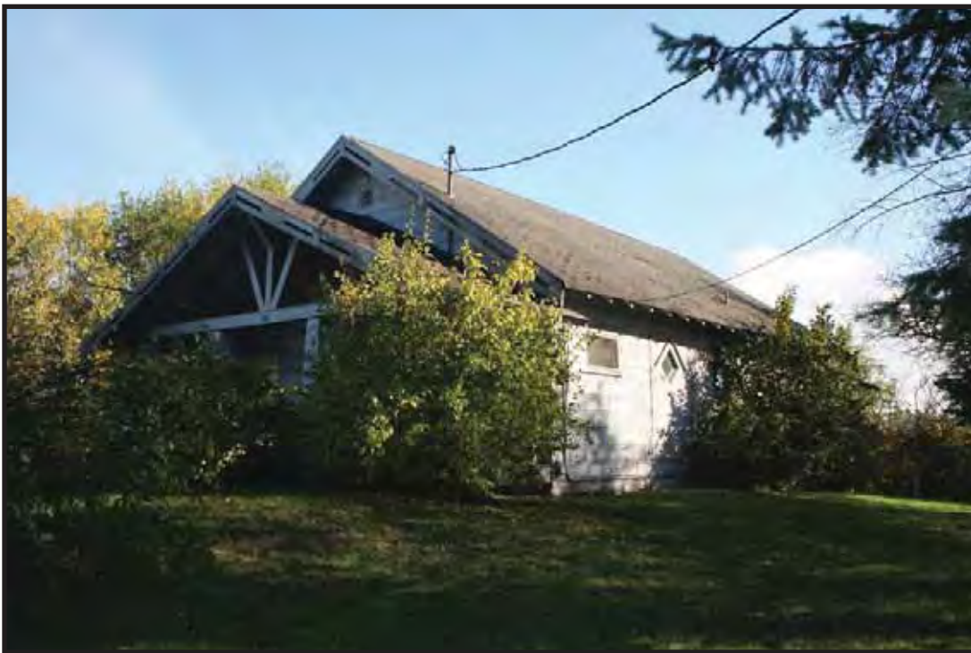
Figure 12. Bean residence, 411 Birch Street, north (front) and west elevations, view to the southeast.
