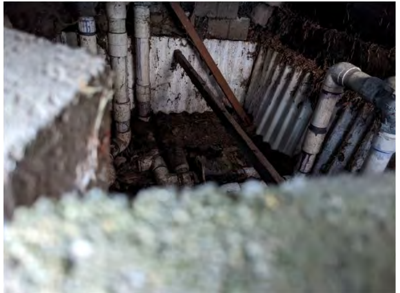
Photo 5 Interior of one of the several subsurface irrigation control structures along the on-site landscaping circles.
