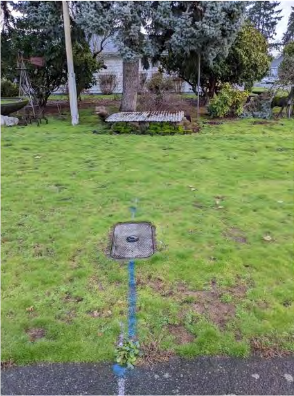
Photo 4 Facing north across a domestic water connection and a subsurface irrigation control structure in the southern portion of the subject site.
