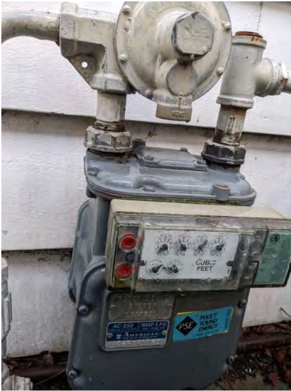
Photo 10 Utility meter at the southwest side of the home.
