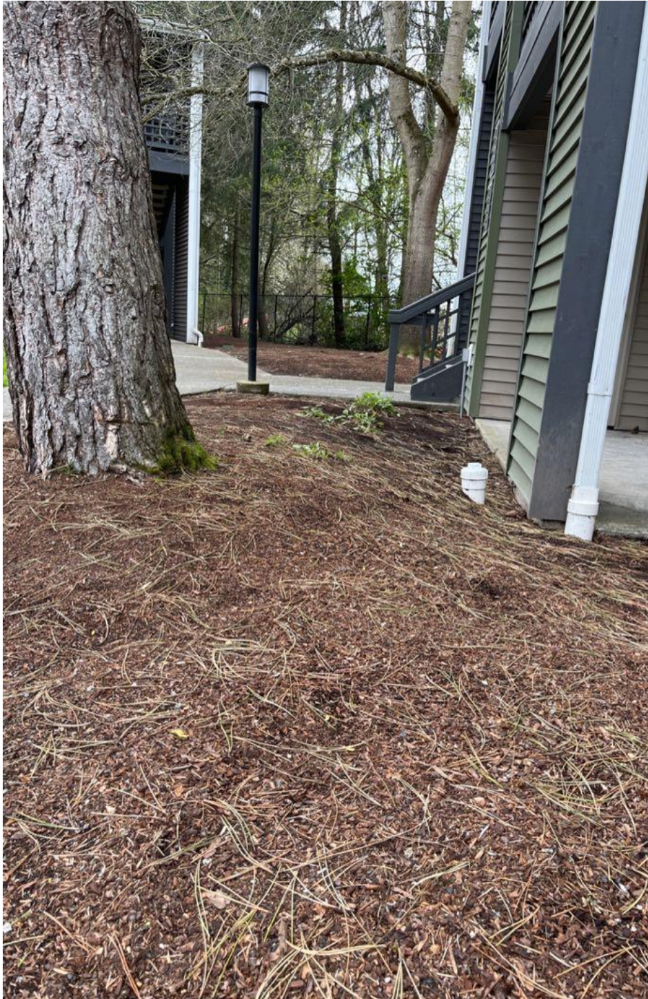
Photo – B Taken 4/20/23. Showing upheaval on tension side of lean on tree #1.
