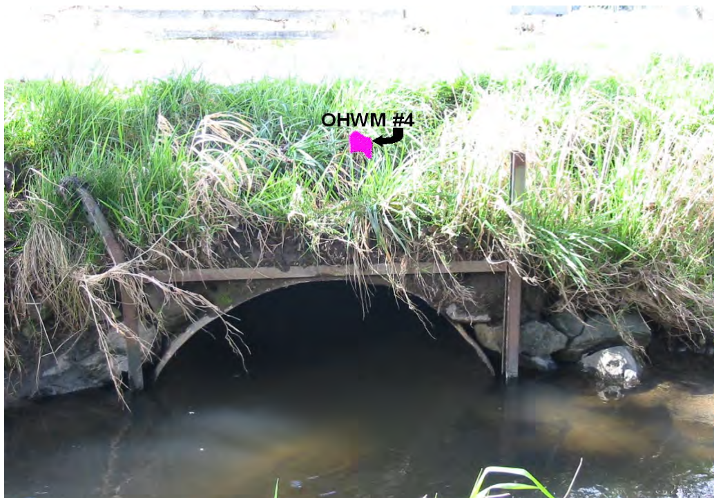
Photo #2: Looking west under an old unused culvert which has been blocked, and no longer conveys water flow to the west under 25 th Street SE. Notice the Ordinary High Water Mark flag #4. (Taken 4/11/08)
