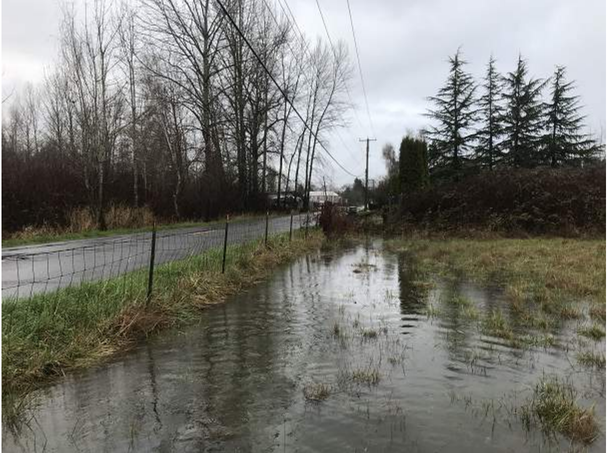
Photo 3. Looking north at the NW site corner during heavy rain event. Stormwater collects in this corner and passes under Freeman Rd within a 12-inch concrete culvert.
