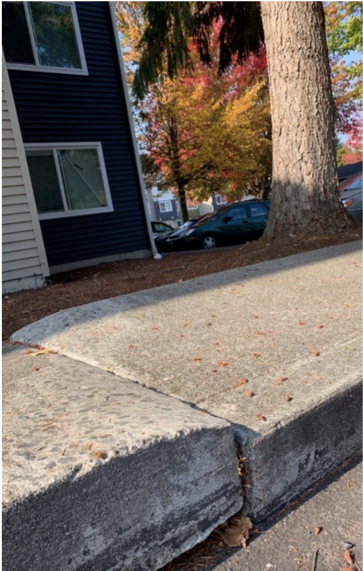
Tree 4: Walk damage & previous surface grinding
