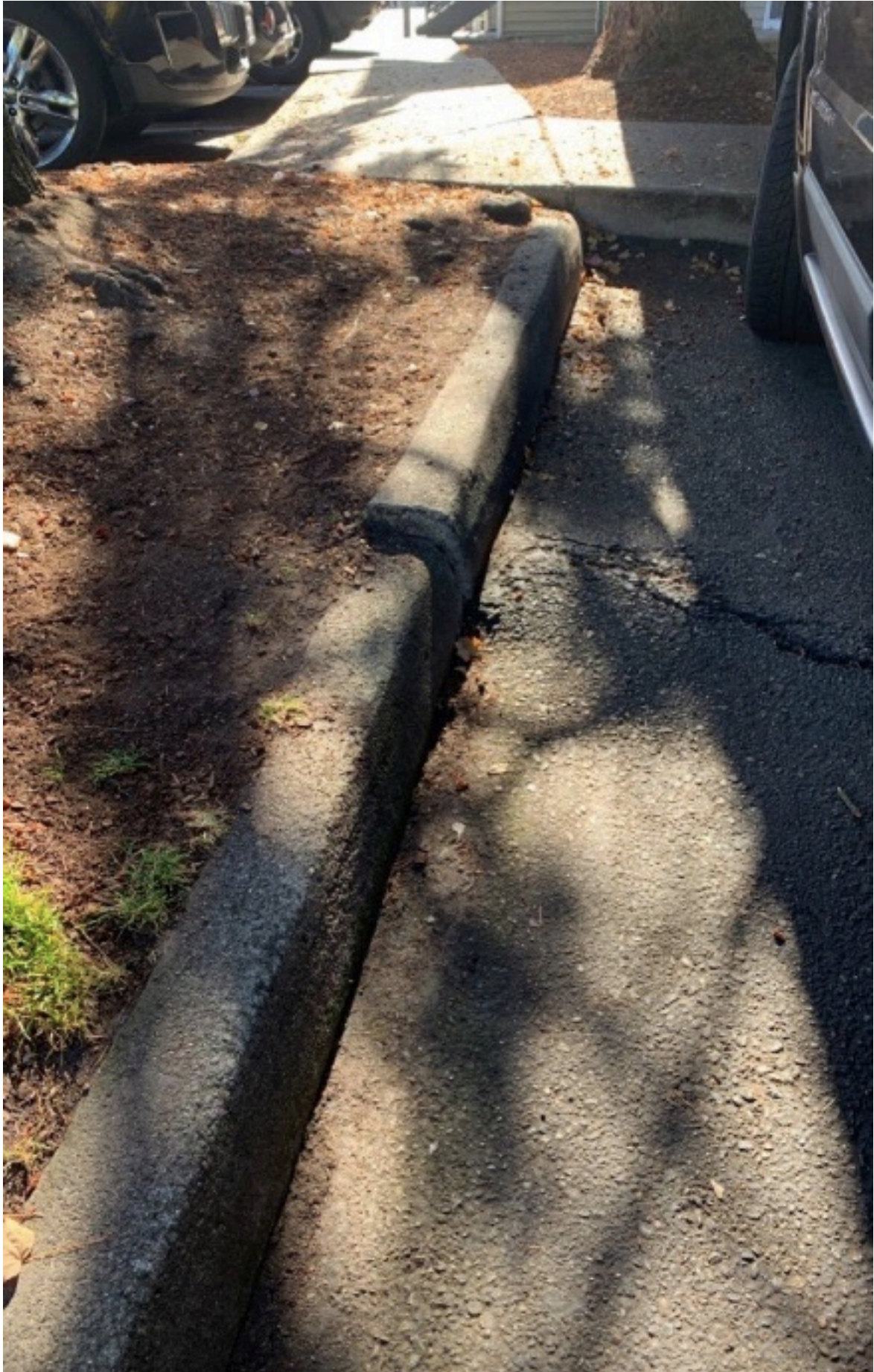
Tree 5: Curb & asphalt damage
