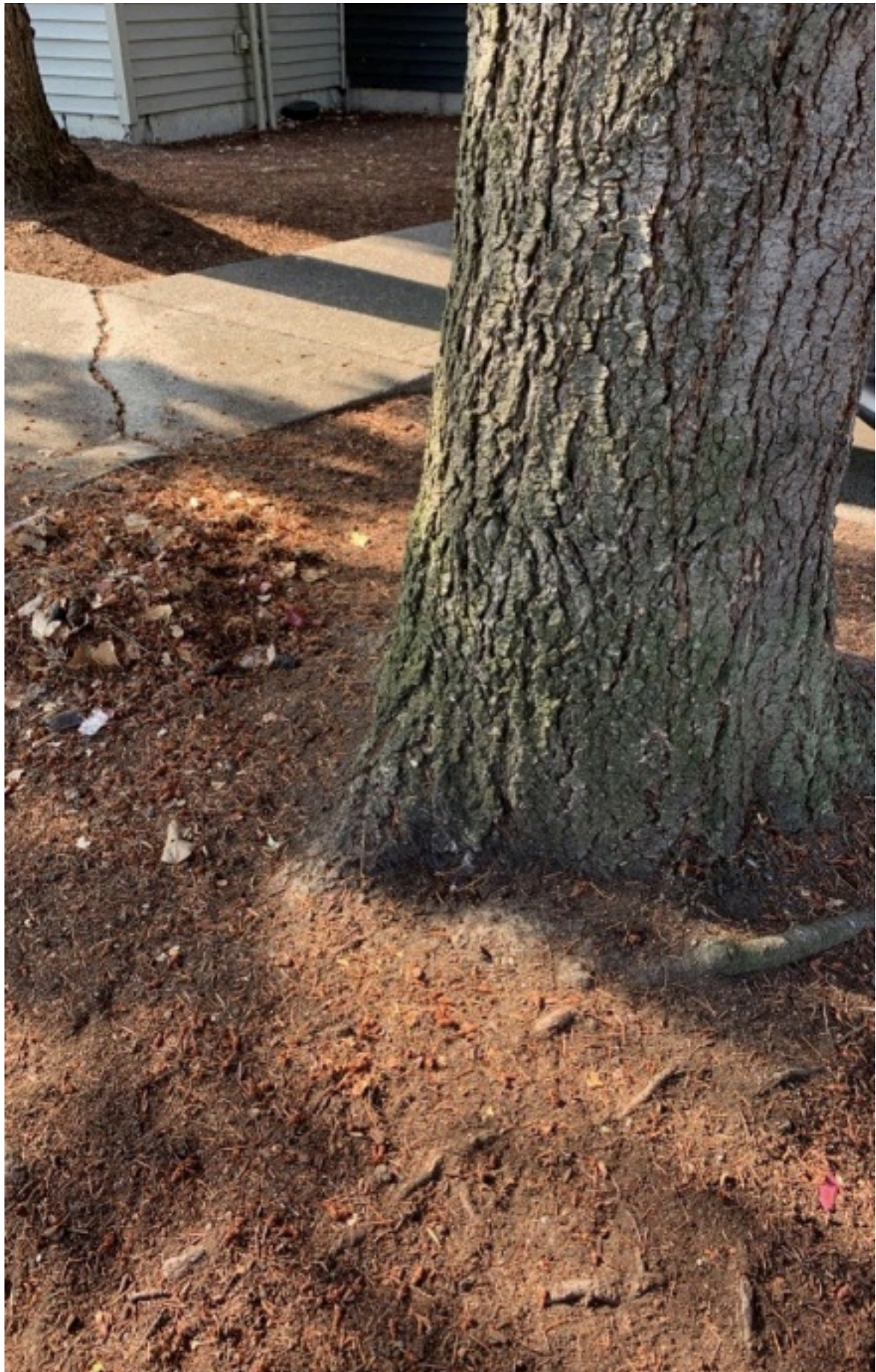
Tree 5: Adjacent walk damage
