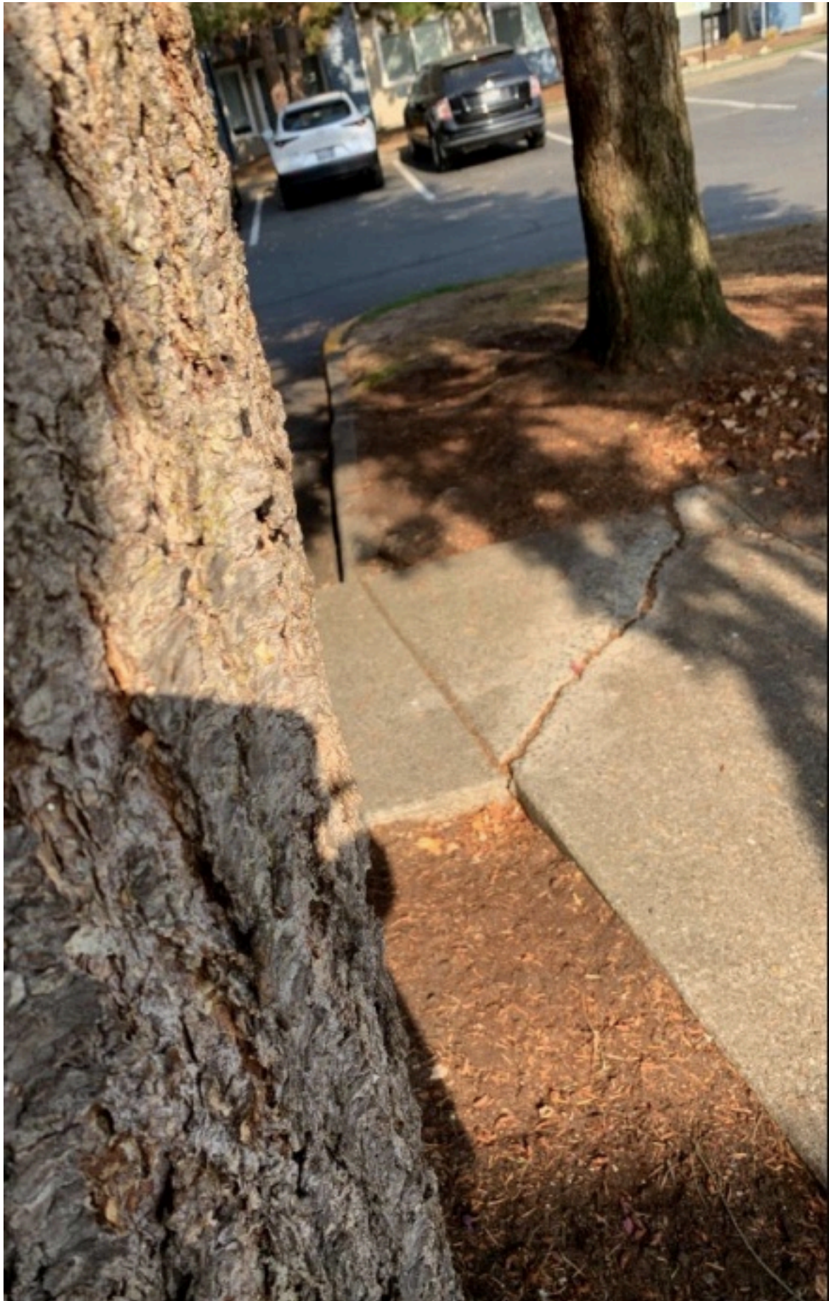
Tree 4: Adjacent walk damage & previous surface grinding
