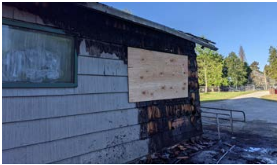
In 2021, the fieldhouse at hit by an arsonist and partially destroyed.
