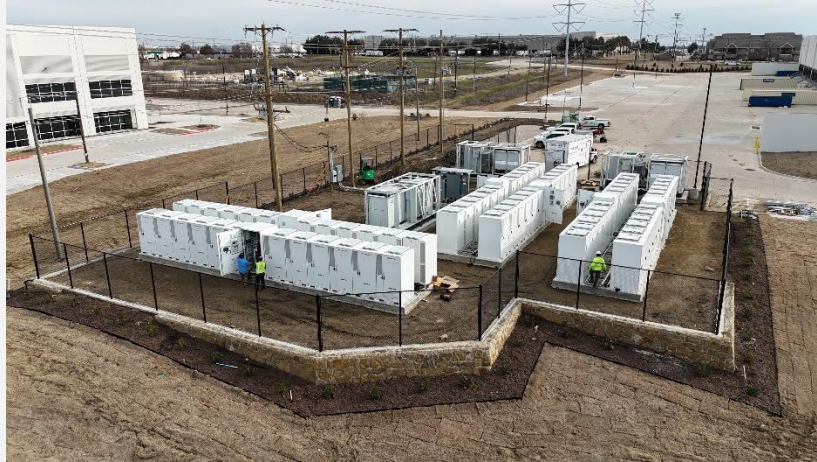
Photo 1. Overview of typical battery energy storage system (BESS) containers.
